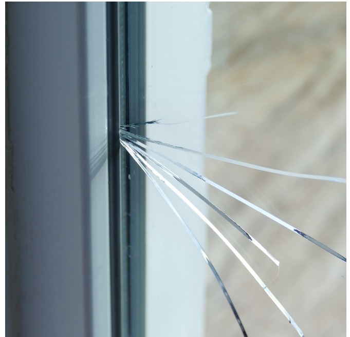
The perpendicular path of the crack starting from the edge of the glass is characteristic of a breakage pattern due to thermal stress.
